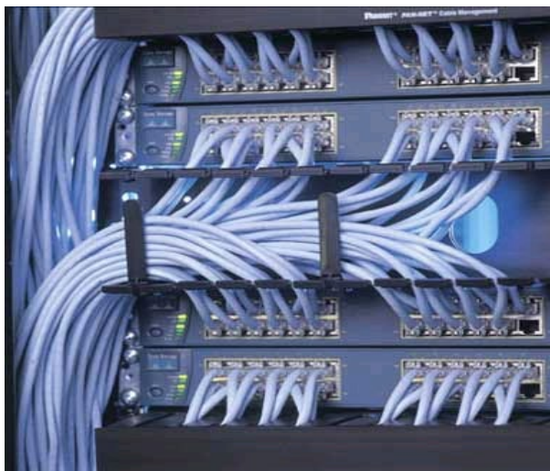
Figure 3.5 – Distribution of Ethernet cables on a panel
