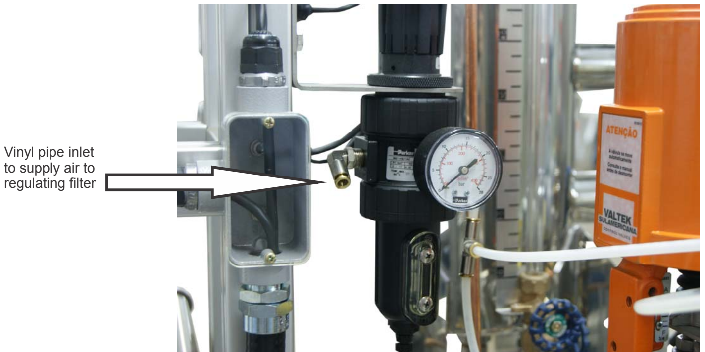
Figure 1.3 – Vinyl pipe inlet to supply air to the regulating filter.
