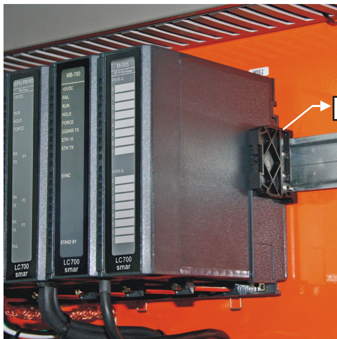
Figure 4.3 – Final post that holds the Racks on rail
